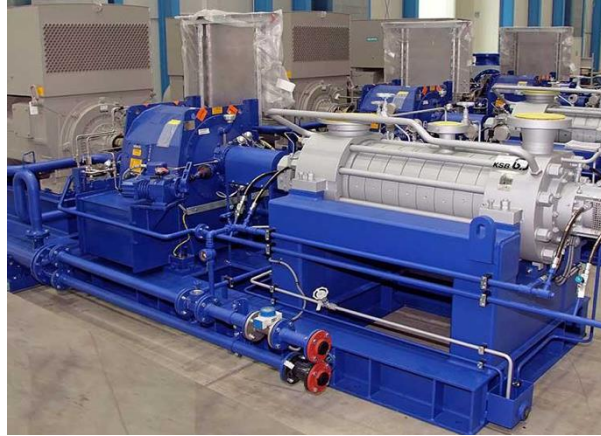
Motors and Pumps
