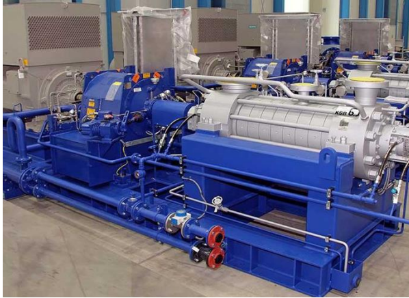
Motors and Pumps
