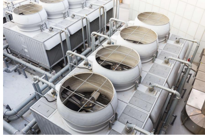
Fans and Gearboxes
